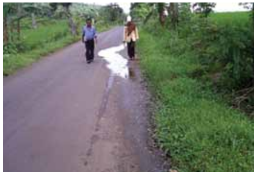
► Inspection of the recently completed Karangsono-Bajulan Road after the rains in Nganjuk district, East Java province.
